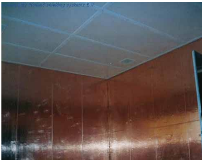
Screened removable ceiling
